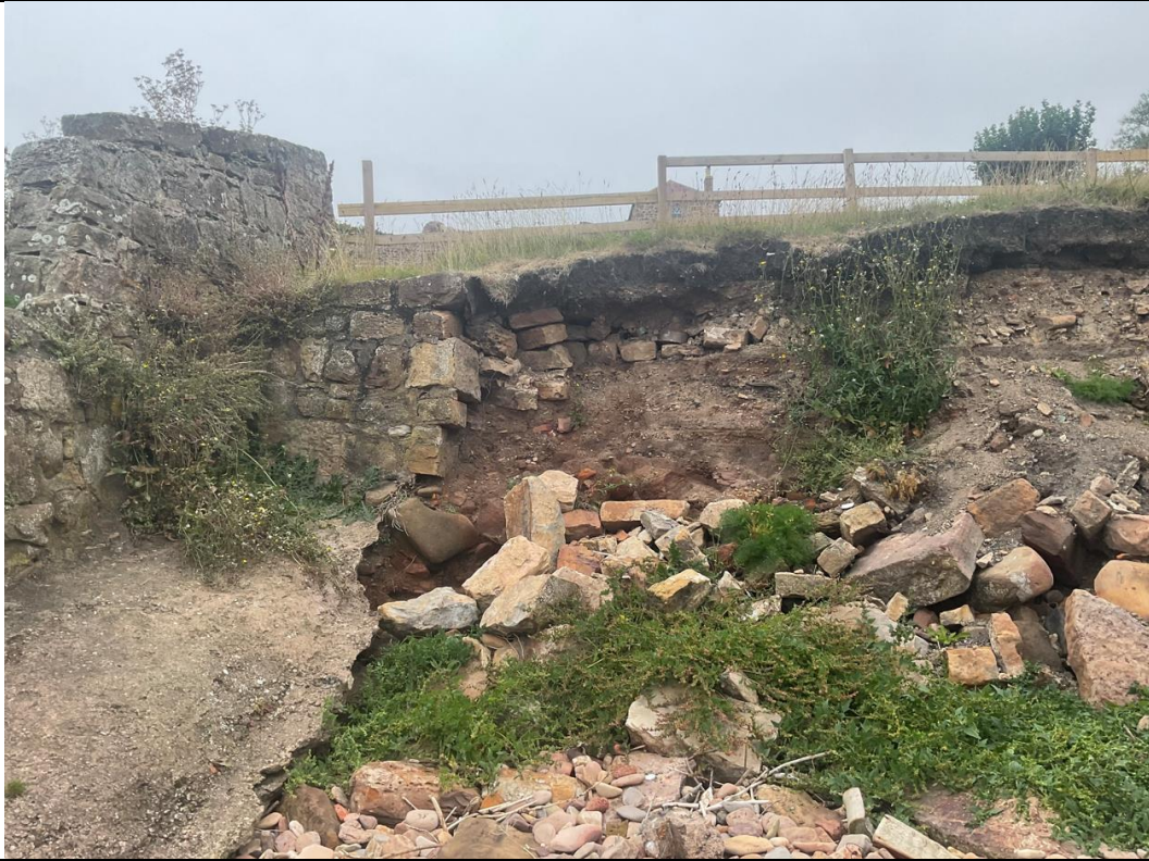
Figure 5- Collapse of the coastal wall taken at approximately ch65.
