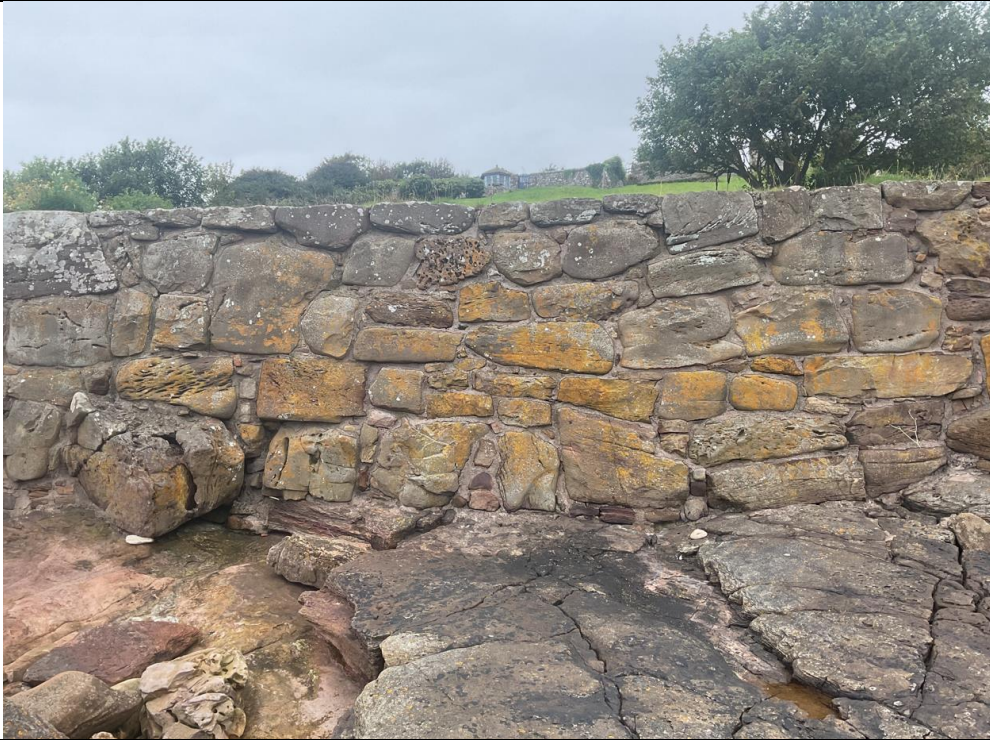
Figure 23- Generally wall condition is good between ch276-297. Larger stone at the base of the wall possibly displaced. Some undercutting to the structure at the base.
