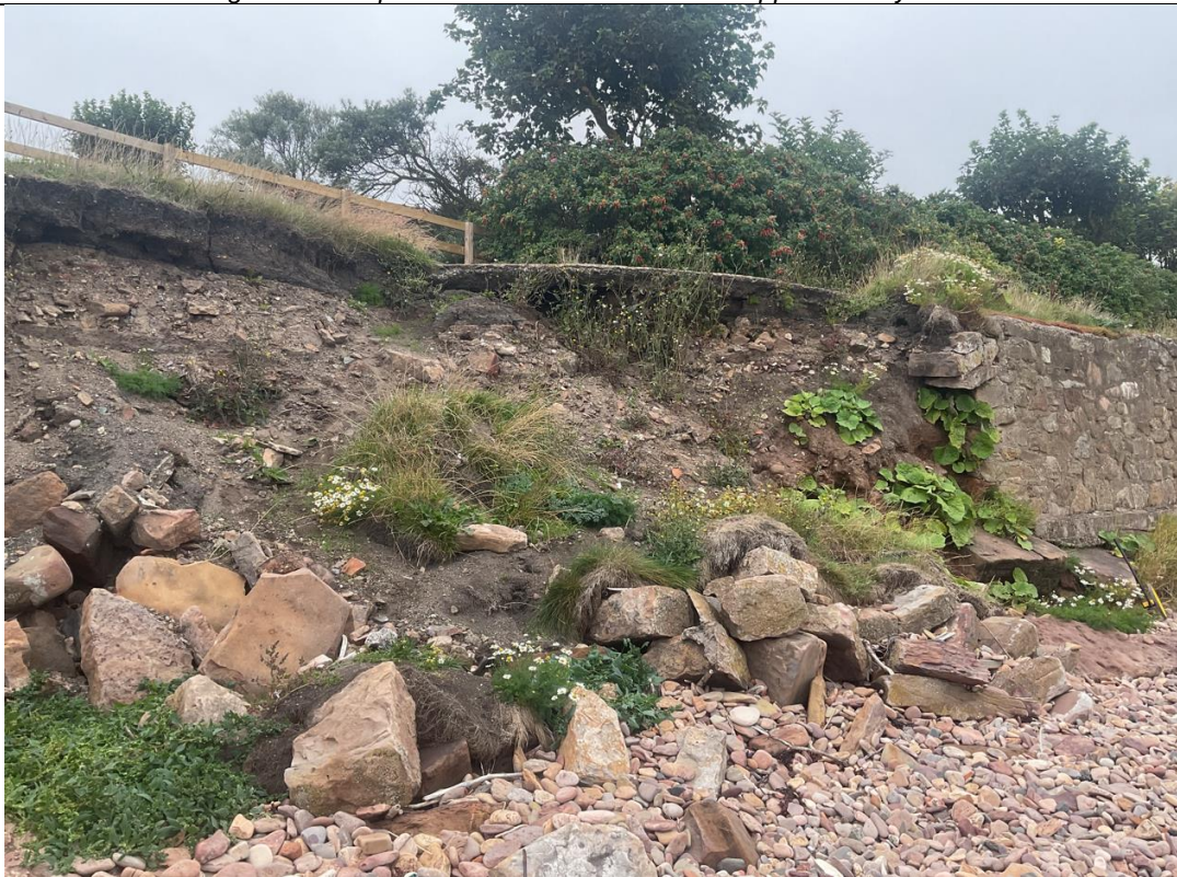
Figure 6- Remainder of the collapsed section from approximately ch65-ch75.
