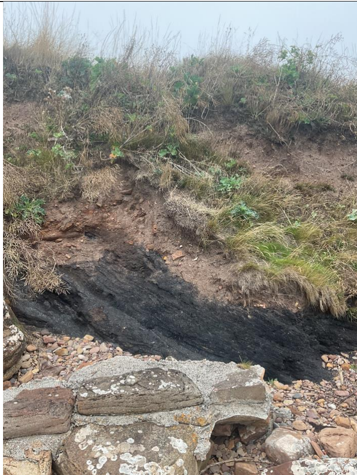
Figure 19- Between ch170-ch239, the wall has been completely eroded. Dark rock exposed, possible coal.
