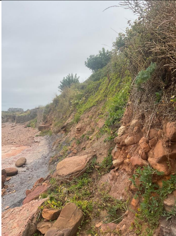
Figure 11- Photo taken between ch85-ch122, wall completely eroded, large mudstone beds visible behind where the previous structure stood.
