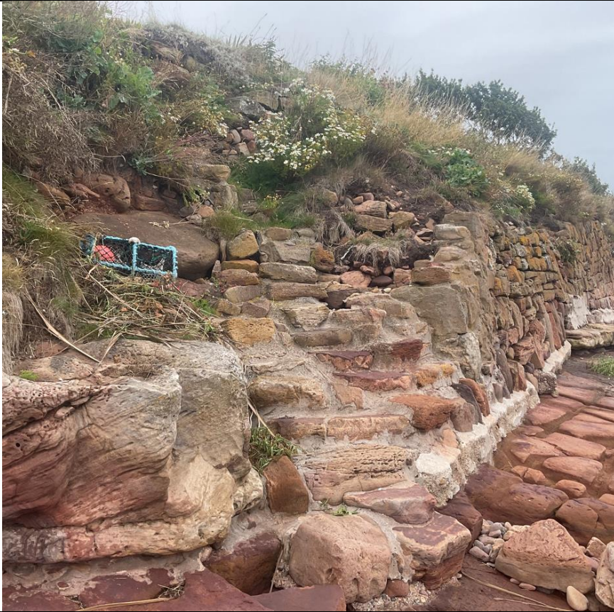
Figure 13- Photo taken between ch122-ch143, wall gradually reappears from the completely eroded state.
