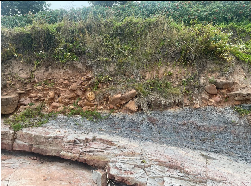
Figure 10- Photo taken between ch85-ch122, wall completely eroded, large mudstone beds visible behind where the previous structure stood.
