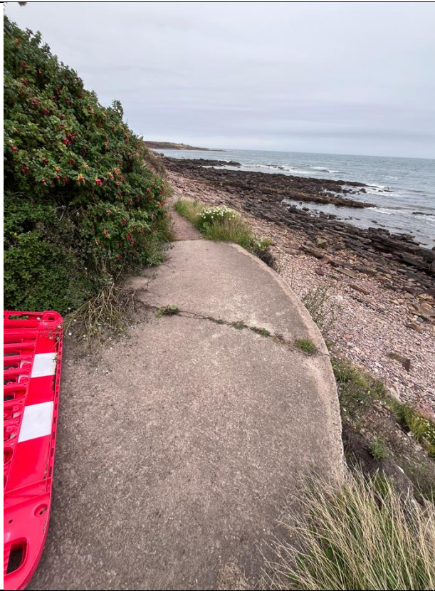
Figure 35- Short 3 metre section between ch65-ch68 of path which is in an okay condition.
