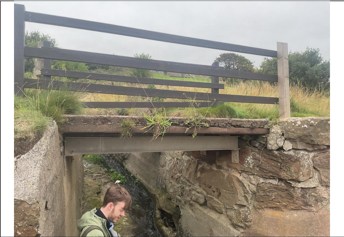
Figure 21- Footbridge located at ch239. Void visible on the northern side of the coastal wall, under the bridge.
