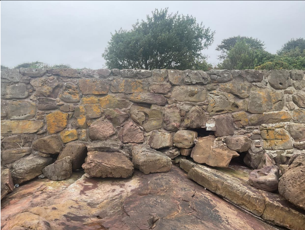
Figure 24- Between ch297 and ch347, mortar and stone condition generally okay. Some stones at the base of the wall possible displaced. Where there is displacement there are voids behind.
