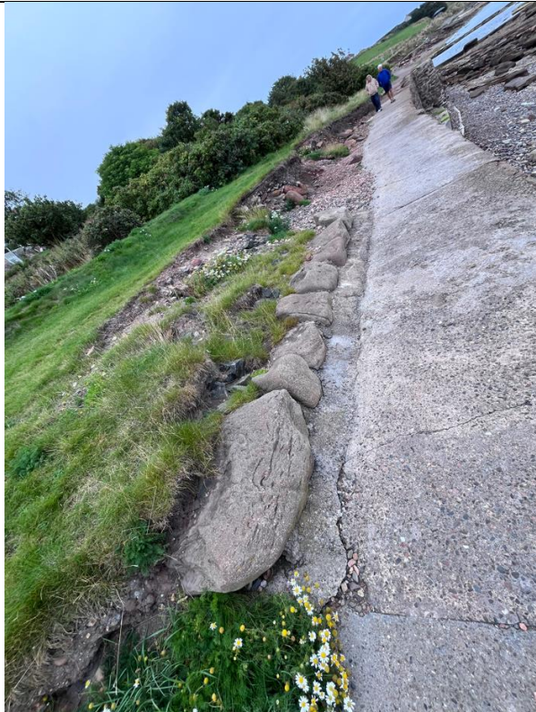
Figure 44- Erosional damage to land west of the path edge, potentially overtopping waves between ch284-ch295).
