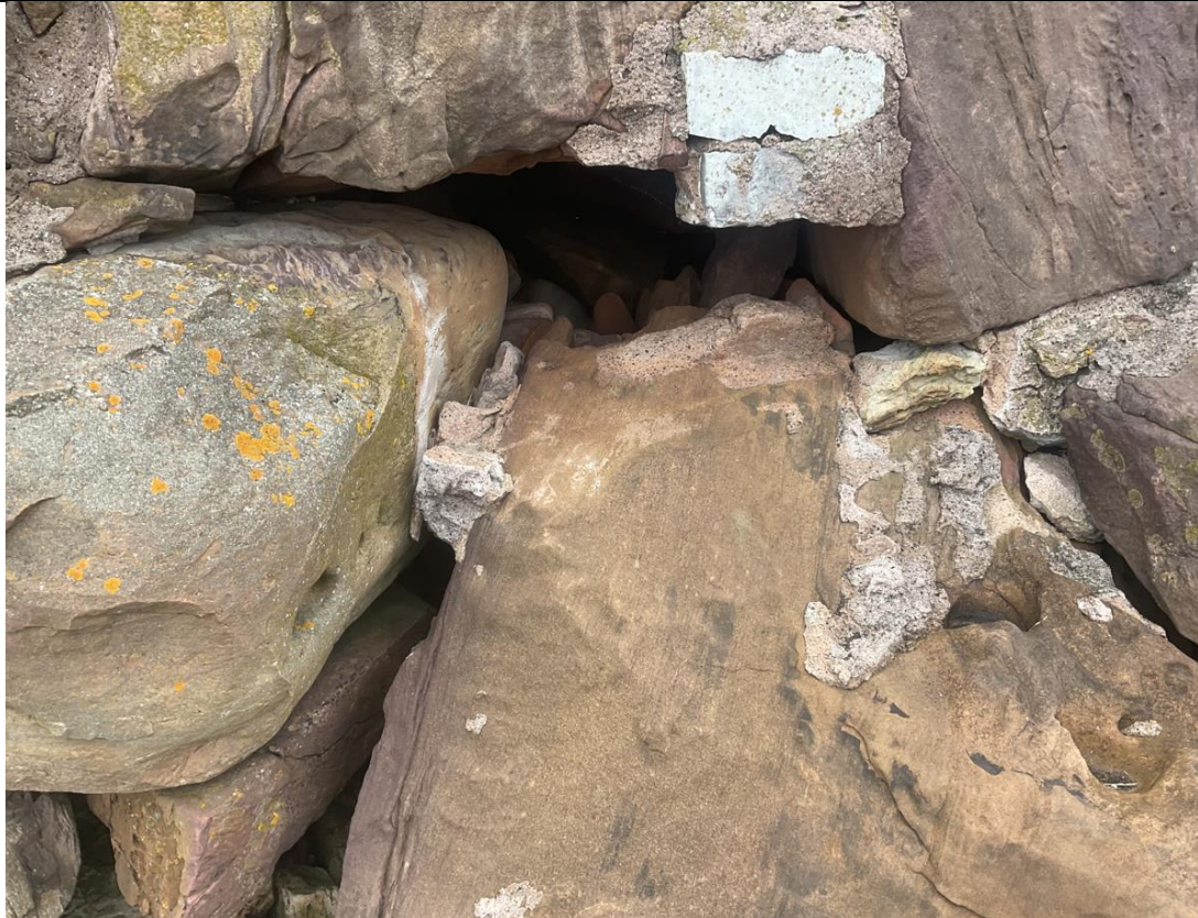
Figure 25- Voids located behind the displaced stones in figure 23.
