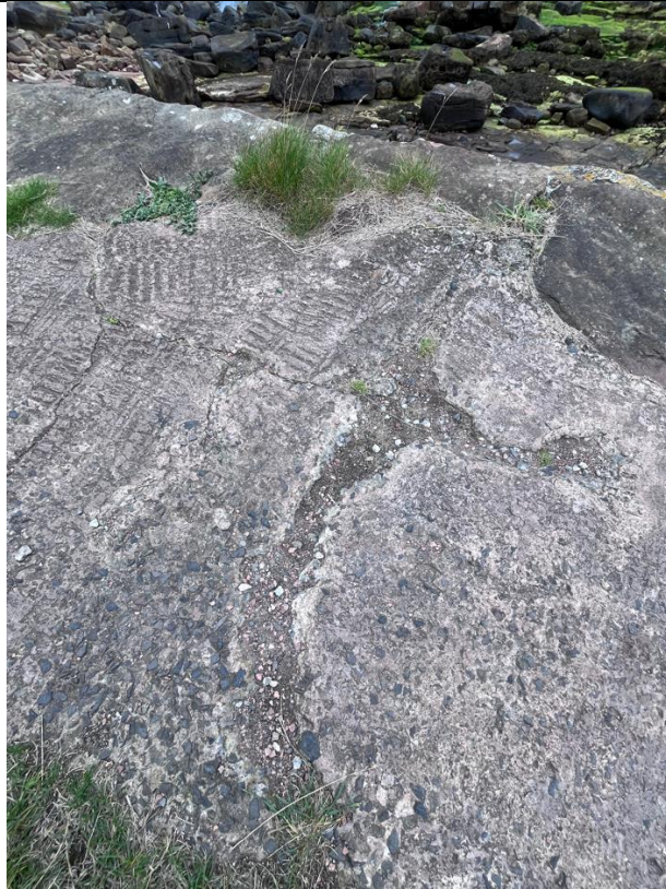
Figure 39- General condition of the path between ch236-ch272. Cracking appears to be over 7.5cm wide, although not altered the structure of the path.
