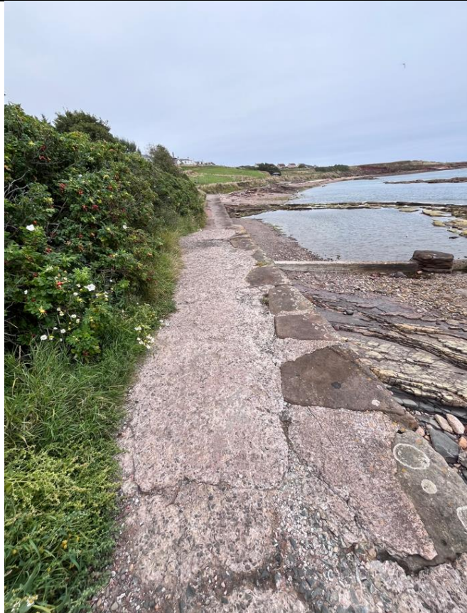
Figure 50- Cracked path surface between ch358-381.8.
