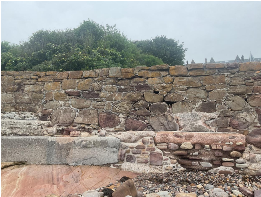
Figure 28- General wall condition between ch347-ch396. Voids located at varying heights u the wall.
