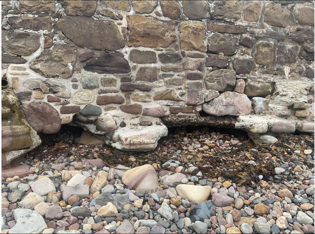
Figure 29- Two areas of undercutting to the wall located between ch347 and ch396.
