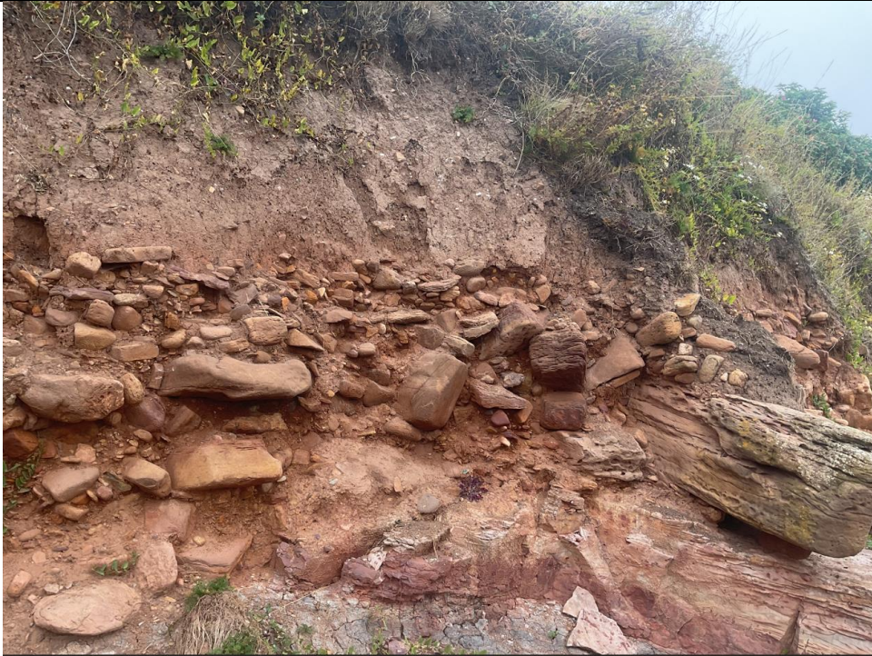
Figure 9- Photo taken between ch85-ch122, wall completely eroded and structural members exposed.
