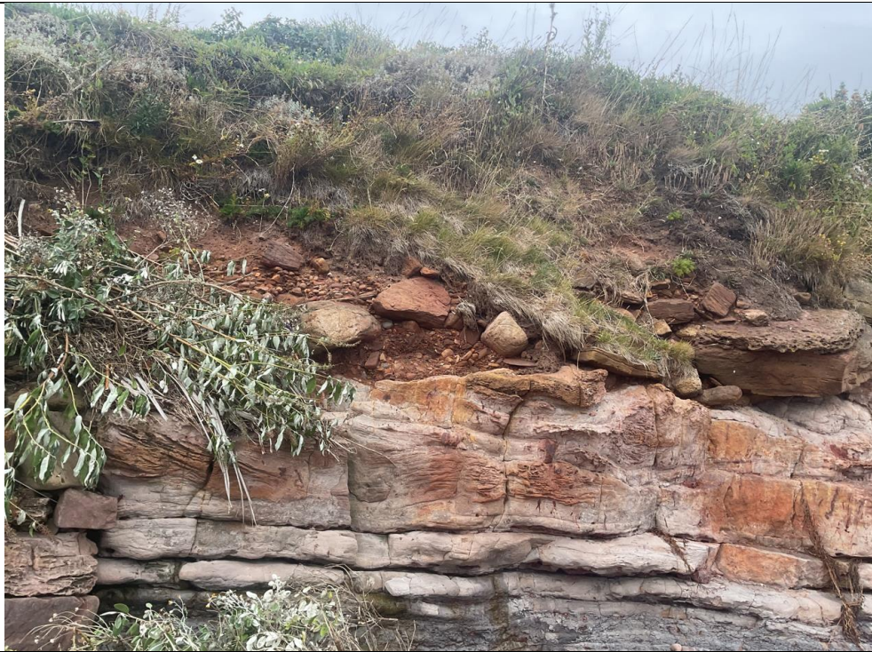
Figure 15- Between ch143-ch149, the wall has been completely eroded and structural members exposed.
