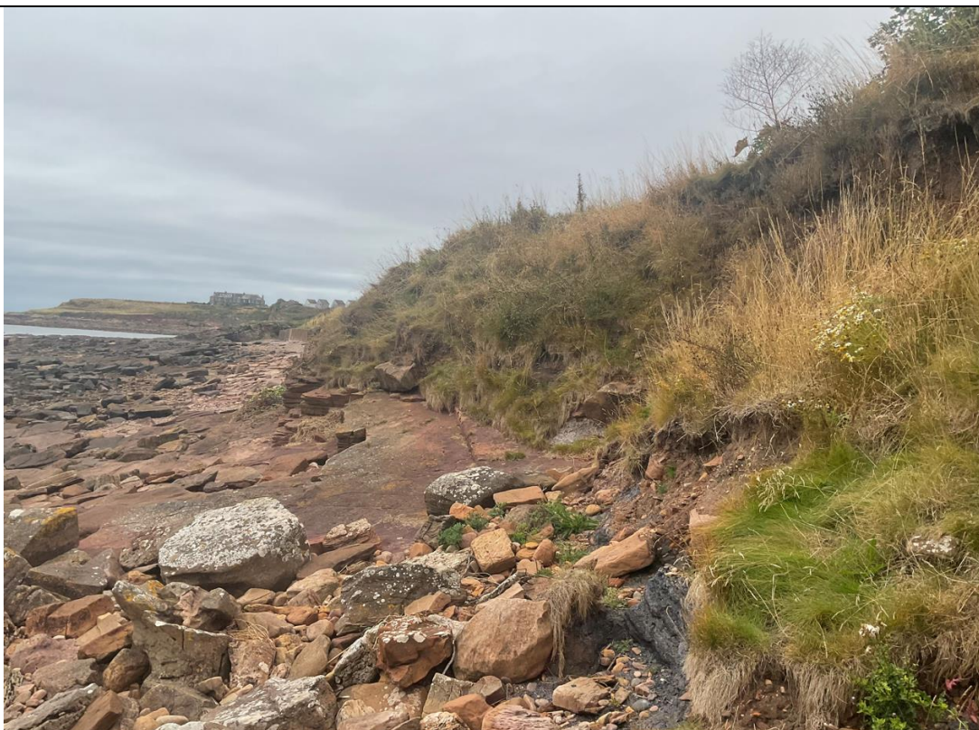
Figure 18- Between ch170-ch239, the wall has been completely eroded. Photo taking standing from the north looking south.
