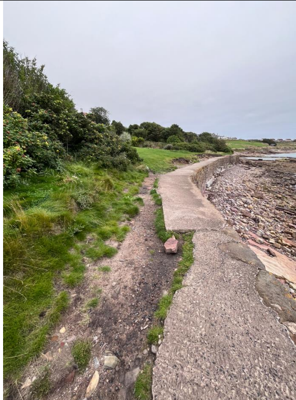
Figure 42- Subgrade materials exposed at the western surface edge, assumed to be subgrade materials. Located between ch284-ch295.
