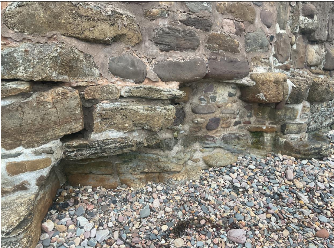
Figure 30- Further erosional damage between ch347-ch396.
