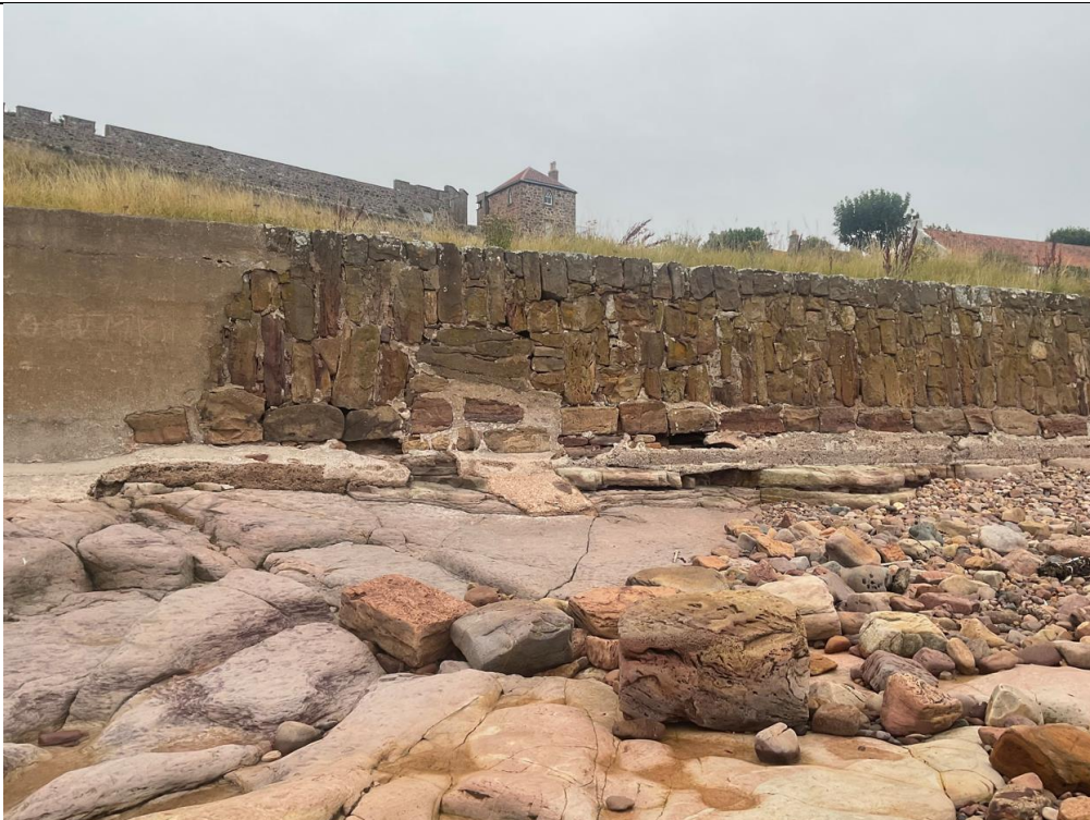
Figure 4- General condition between ch23.5-ch65. Mortar erosion and significant undercutting to the concrete foundations.
