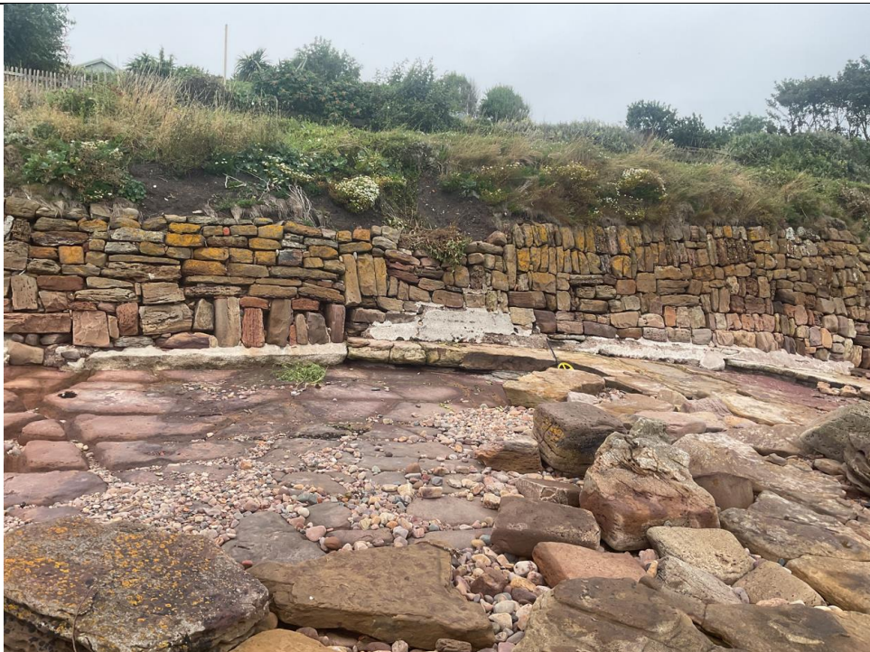
Figure 14- Frontal view between ch122-ch143, complete absence of mortar concrete foundations see, okay. Where the wall has been founded on a large sandstone bed there has been undercutting.
