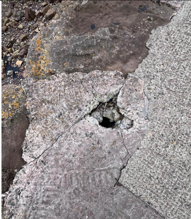
Figure 49- Area of surfacing missing between ch349-ch358.
