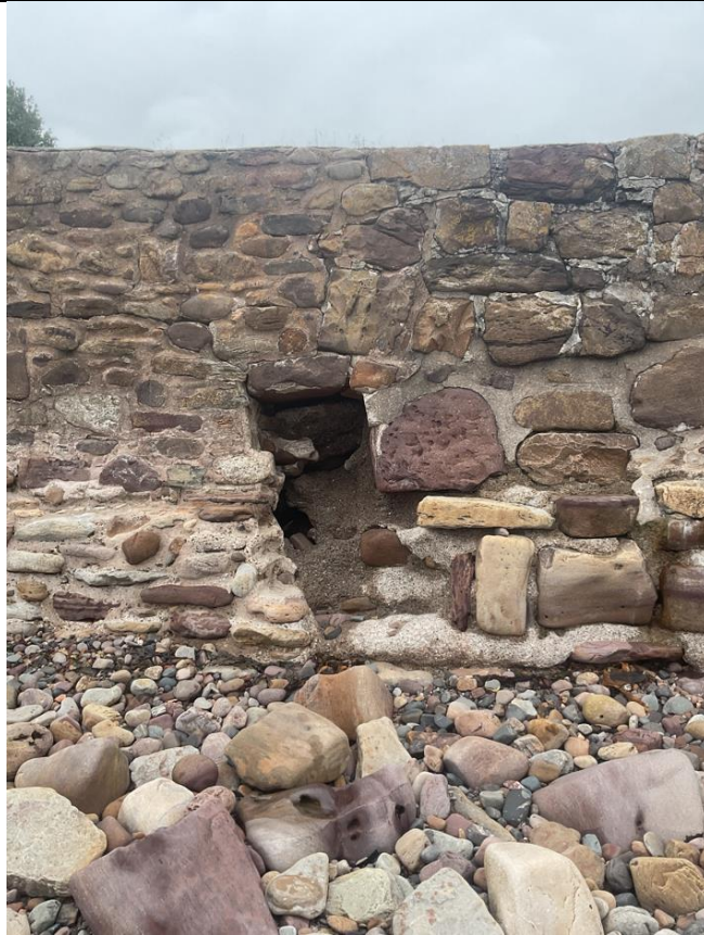
Figure 27- Large void located between ch347-ch396.
