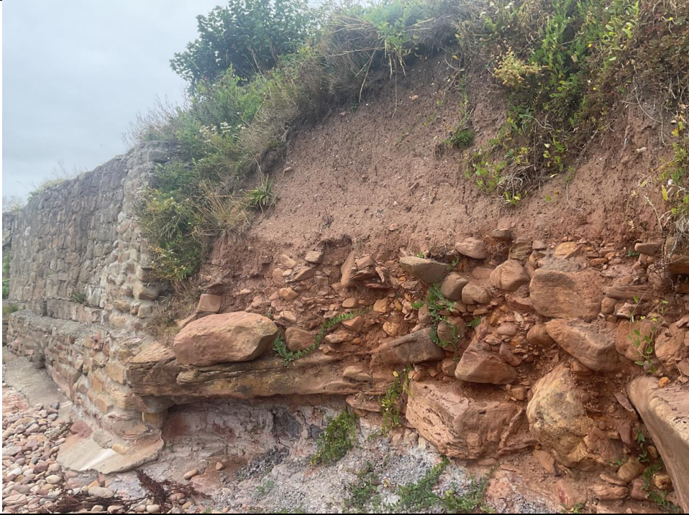
Figure 7- Section of wall standing between ch75-ch85. Photo taken from the north side of the damaged section looking south.
