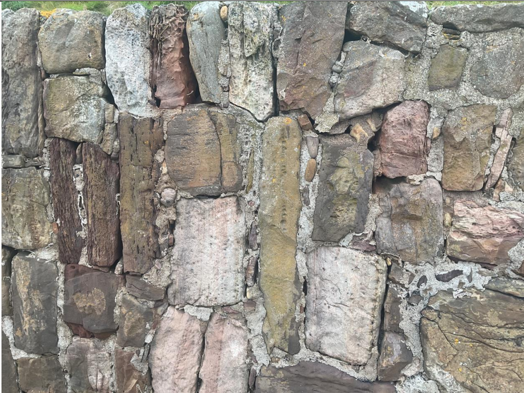
Figure 2- Closer condition of weathered stones and mortar representative of ch000-ch23.5.
