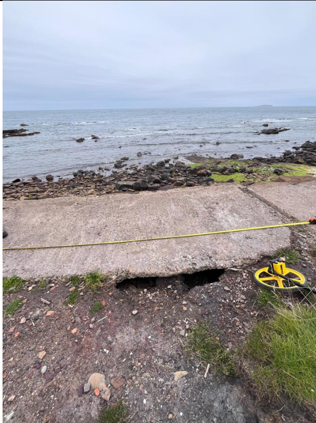
Figure 43- Large void at the western edge of the path located at approximately ch295.
