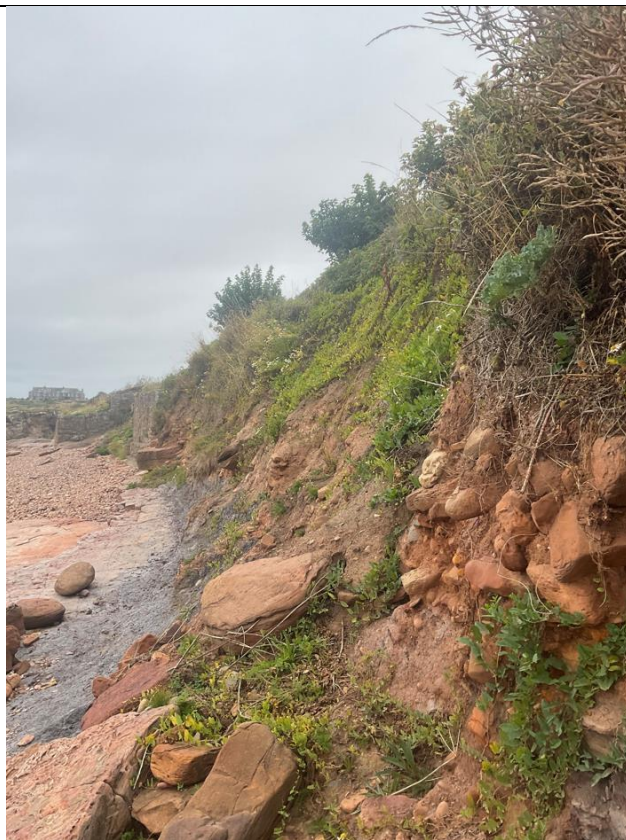
Figure 12- Photo taken between ch85-ch122 facing south, wall completely eroded, near vertical slope.
