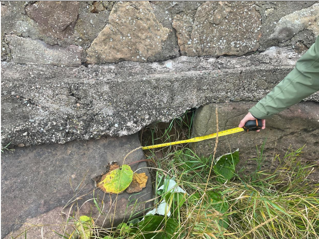
Figure 8- Undercutting to the concrete foundations of the wall located between ch75-ch85.
