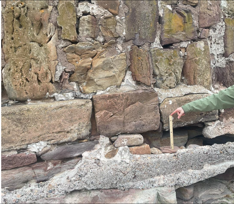
Figure 3- Undercutting of concrete foundations between ch23.5-c65.
