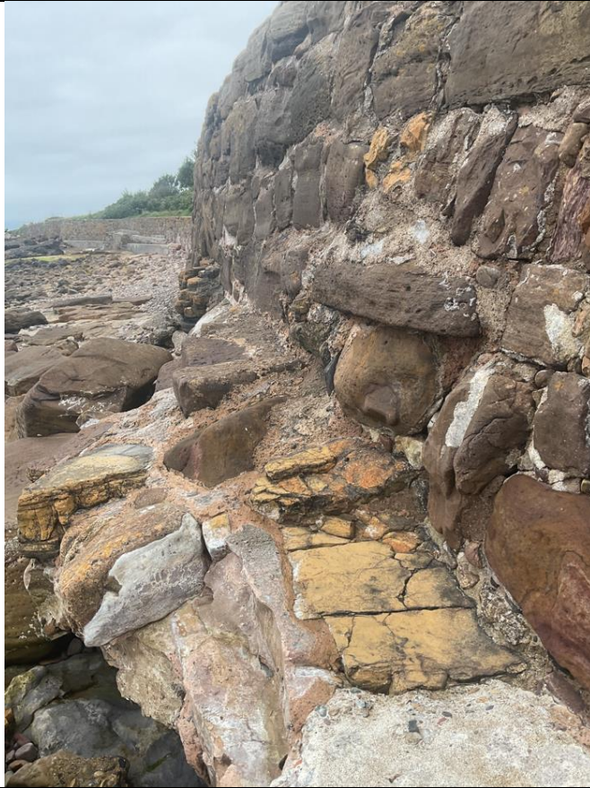
Figure 31- Significant displacement of stones at the base of the wall located at ch393.
