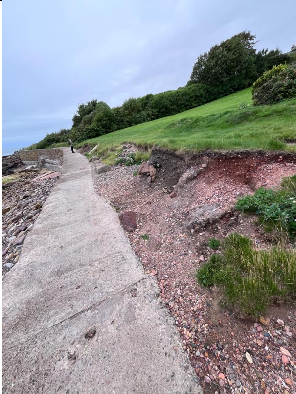
Figure 45- Erosional damage to land west of the path edge, potentially overtopping waves between ch284-ch295).
