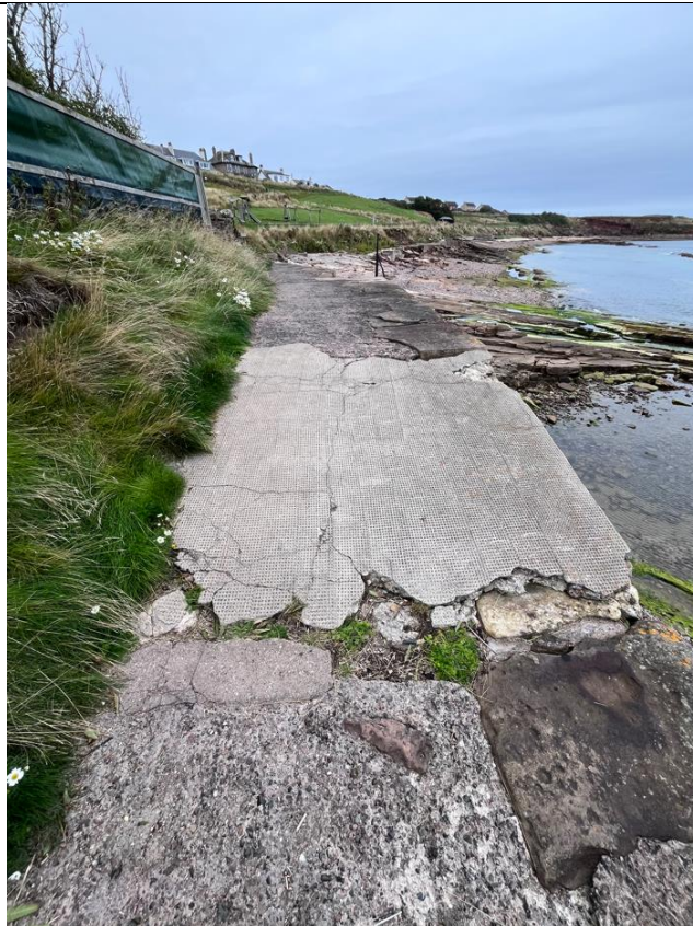
Figure 54- Damaged ramp/slope to lower area of coastal path located at approximately ch414.
